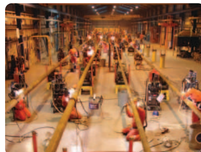
Welding 4" and 6" inner pipes prior to being pulled into the sleeve pipe
