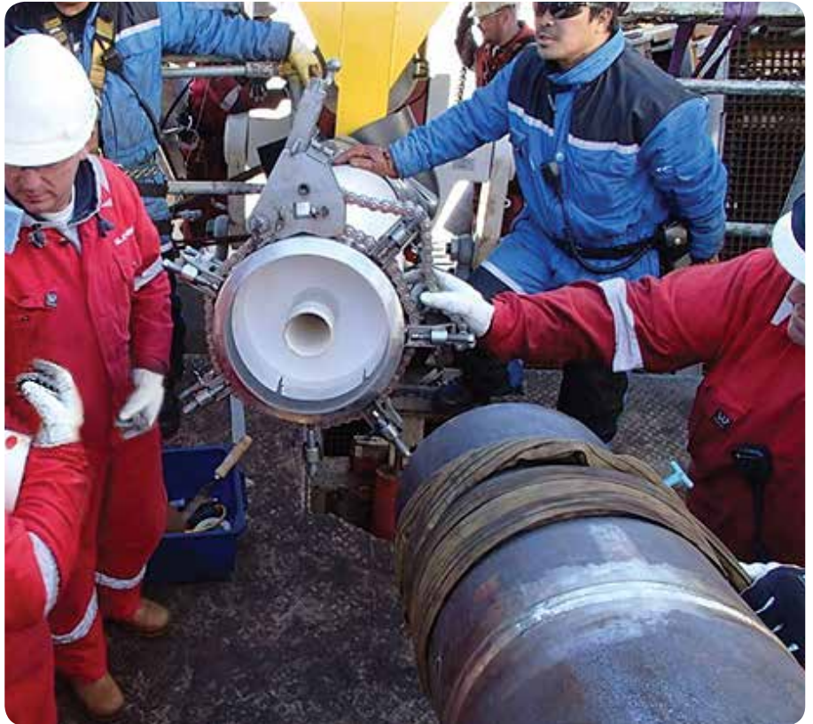
By-pass purge enclosure in place
