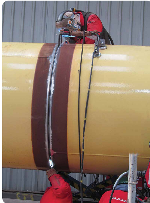
56-inch Bundle carrier pipe
