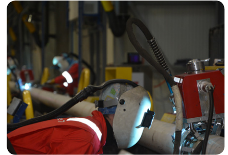
A total of 112km of pipe will be welded on the Catcher project
